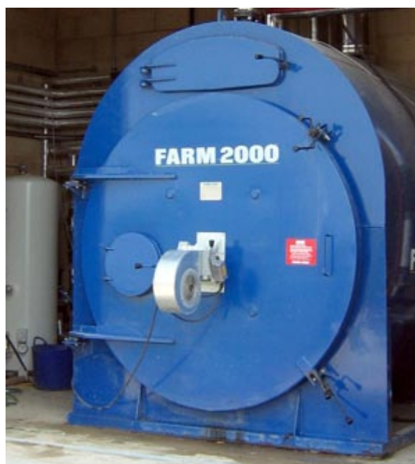
Figure 2 Big bale burner / boiler 13
