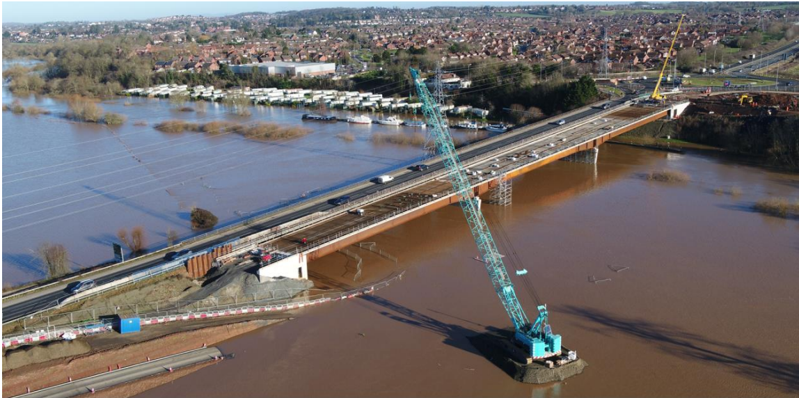
A4440 SLR4 Flood Event during construction
