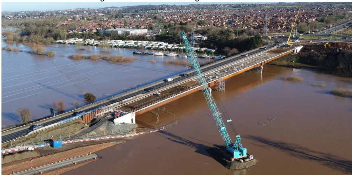
Figure 11-3 – Flood event during SLR4 construction
