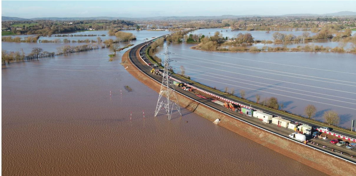
Figure 11-2 – Flood event during SLR4 construction
