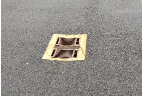
Picture 4 – this drain has been highlighted to reduce the risk of tripping.
