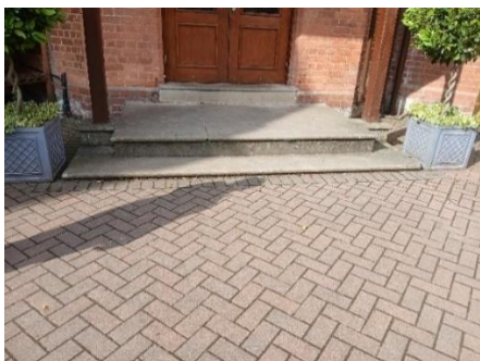
Picture 8 – doorsteps need to be marked up with a colour that contrasts easily with the tread. Doorstep edges/nosing to all buildings need to be colour contrasted in hard wearing paint.
